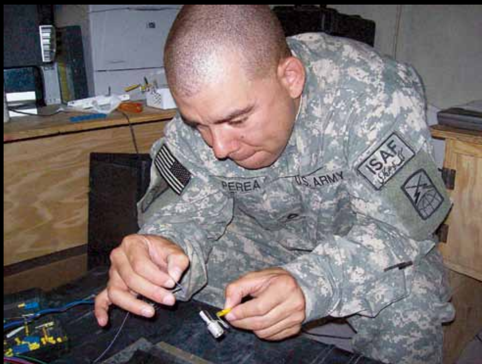
SFC Alexander Perea, HHD 43rd Signal Battalion, terminates a fiber optic cable to provide telecommunication for the the Jalalabad TCF facility in Afghanistan May 2009.
