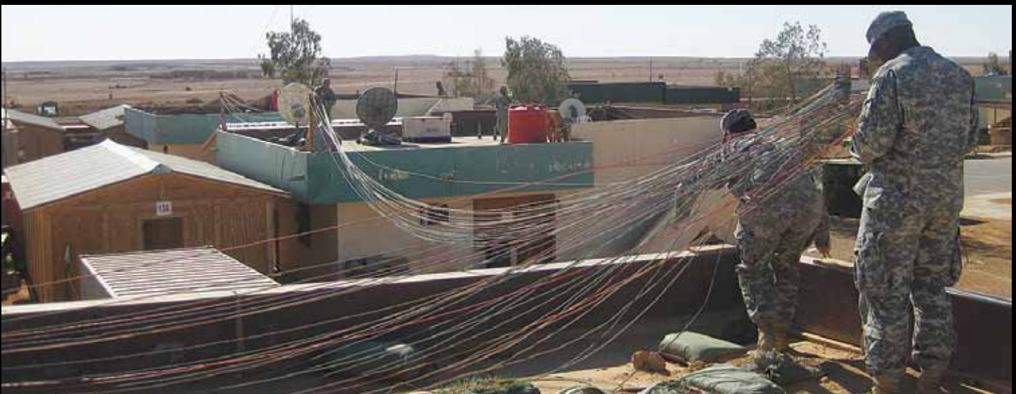
Cable dawgs under the command of 1LT Brandon A. Eicher rearrange and test NIPR and SIPR CAT-V wire around the TCF of Camp Korean Village in November 2009 after a sandstorm damaged cables across the post.
