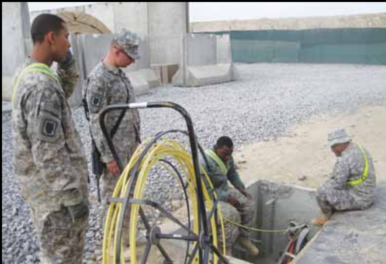
Members of the 57th Expeditionary Signal Battalion lay fiber optic cable at U.S. Air Force Camp Davis January 2010 to provide connectivity to the aviation brigade at Kandahar Airfield.
